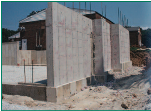
Construction is well under way at 1701 White Columns Drive, where the foundation was completed over the summer.
