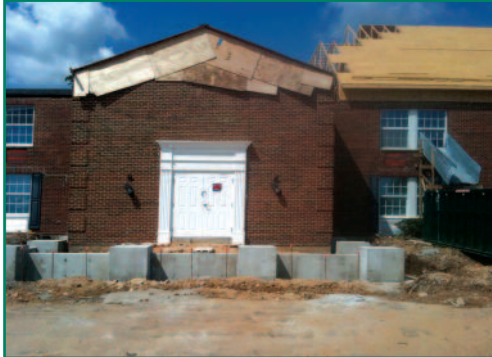
Stop by the construction site over Homecoming on October 2 at 11 a.m. to take a tour and see the progress on the house.
