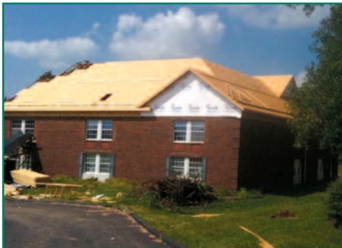
Much progress was made this summer, including the installation of the roof trusses.
