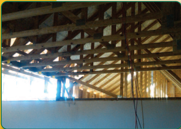
The roof has been raised already and the drywall started in mid-January and parking lots started in November.
